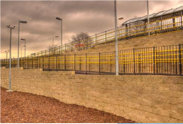
Anchorage Alaska: 3,500m 2 of modular block retaining wall for a rail road embankment. Maximum wall height 5m.
